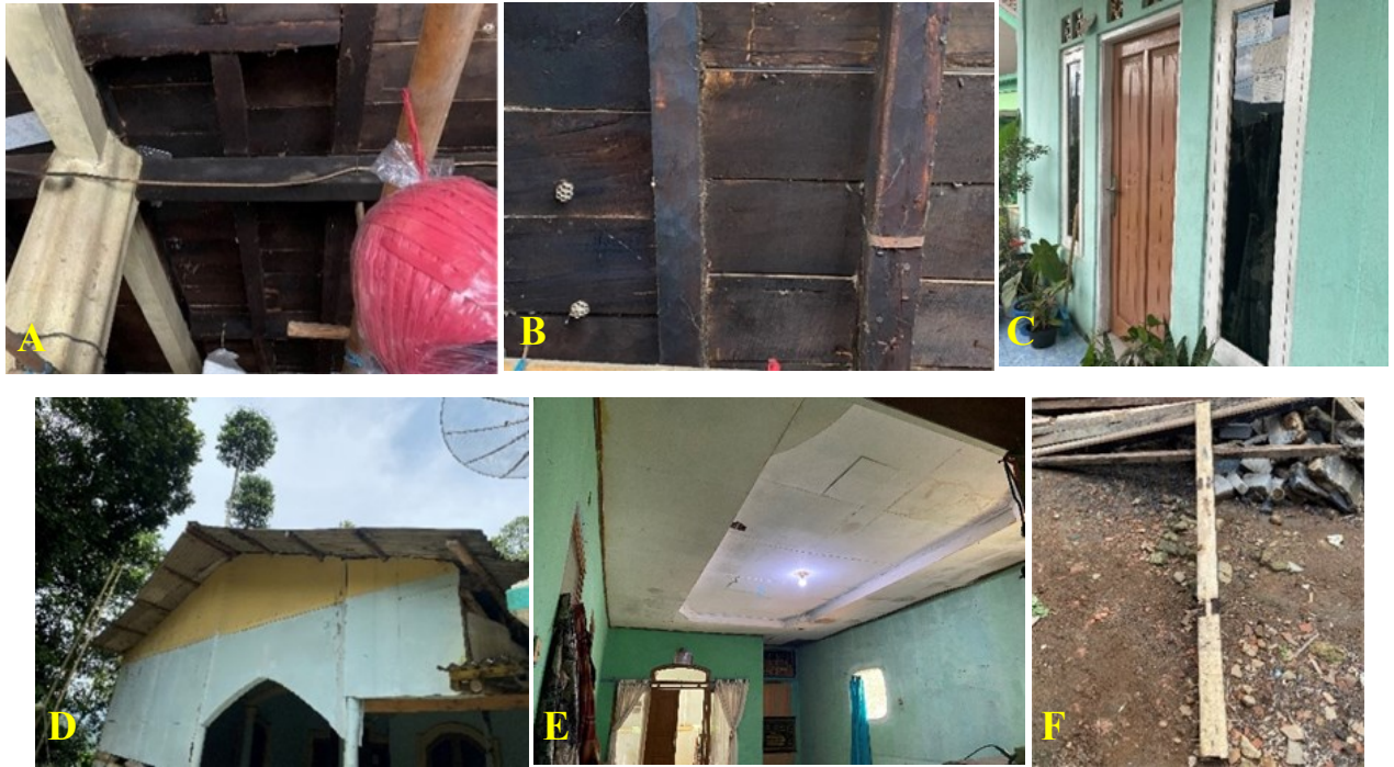
Fig. 3. The utilization of C. argentea and C. tungurrut wood. A & B. Castanopsis argentea wood is used for house ceilings. C. Castanopsis argentea wood for window frames. D. Castanopsis argentea wood for casings. E & F. Castanopsis tungurrut wood is used for roof rafters. Photos by Elbibiya Izzul Penidda.
